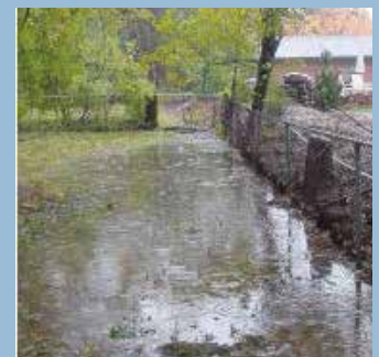
Blocked Drainage Swale
